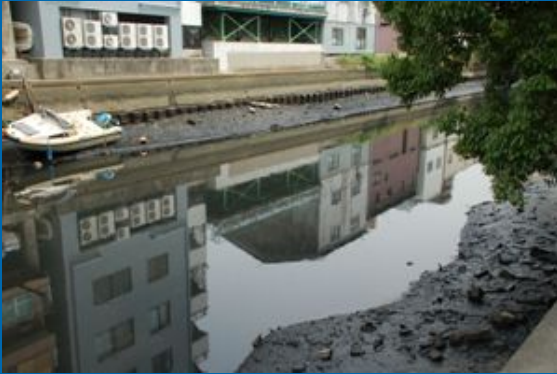
Sludge is appearing around the Gojo Bridge Photo by NIT River Survey Group
